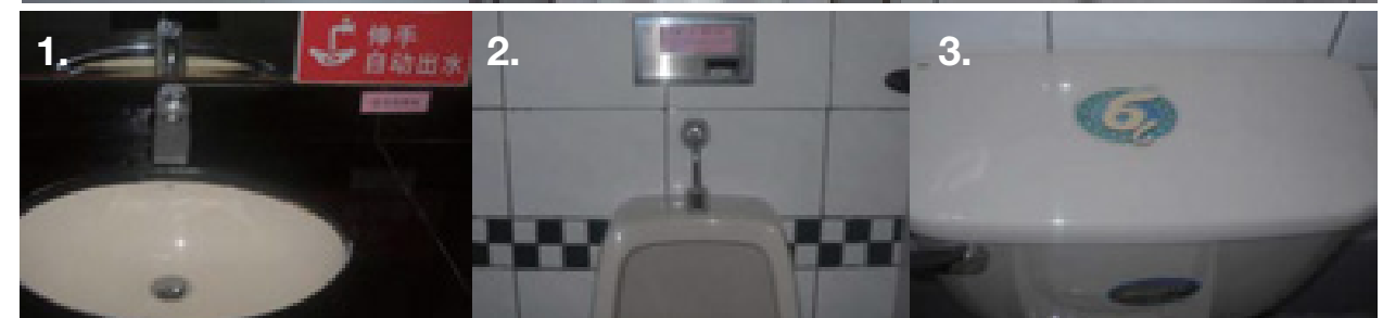
1. Install water faucets with auto on-off sensor. (Photo: Kunshan) 2. Install urinals with auto-flushing infrared sensor. (Photo: Kunshan) 3. Install water-saving toilets. (Photo: Kunshan)
