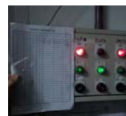
Ventilator capacity concentrated in the 19:30-07:30 period. The OFF record sheet is also shown here.
