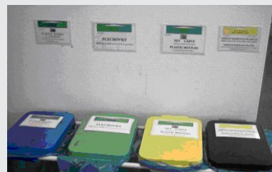
In offices, canteen and locker rooms there are both types of waste: separated (plastic bottles, plastic cups from coffee machine and drink cans) and mixed communal waste.
