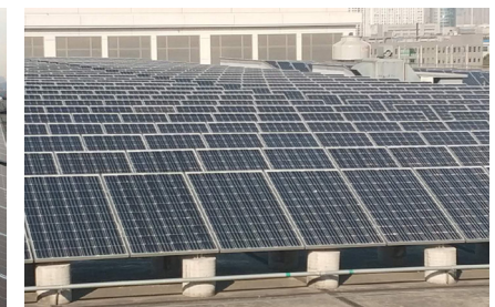
• Solar panels in the Kunshan OPT Plant
