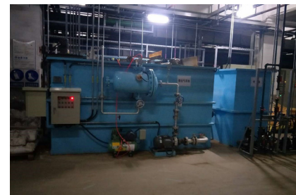
● Kunshan OPT Plant - Exterior of the wastewater treatment station
