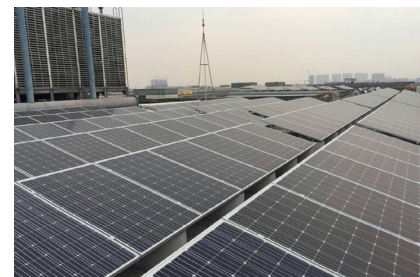
• Solar panels in the Zhongshan Plant
