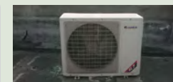
Installed ventilator in office areas to avoid using central air-conditioner during holidays.
