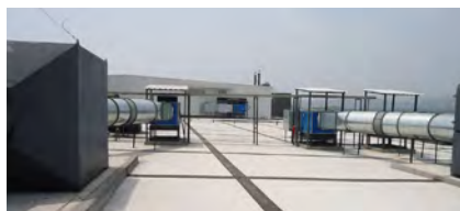
Chongqing Plant - Set the large equipment room at the building's top floor.
