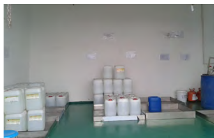
Chongqing Plant - Measures of leakage prevention in explosion-proof chemical storage room.
