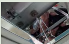
Added pull switch to lights and the staff were asked to turn off the lights when leaving their seat so as to reduce waste.
