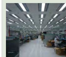
Adjusted ceiling grid lamp.
