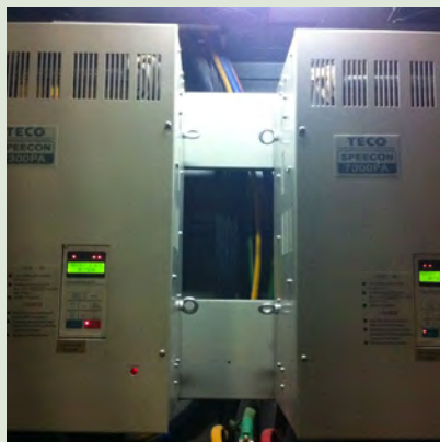
Variable-frequency control of Air-conditioner chiller.
