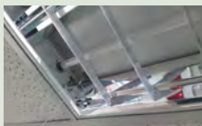
Substituted T8 lighting tubes with the T5 type.
