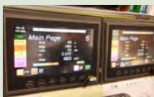
Introduced the electricity monitor system.
