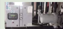
Added variable-frequency control to the air-conditioner in the warehouse to achieve automatic temperature control.
