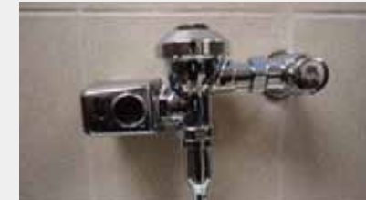
WMX Site installed wash basins with an integrated proximity flush system
