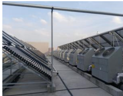
● WKS_Solar/air-source heat pump hot water system for Dormitory
